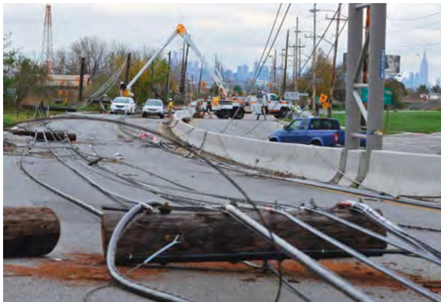
MULTIPLE CREWS from New Jersey’s Public Service Enterprise Group fix poles and downed lines to restore power after Hurricane Sandy.
