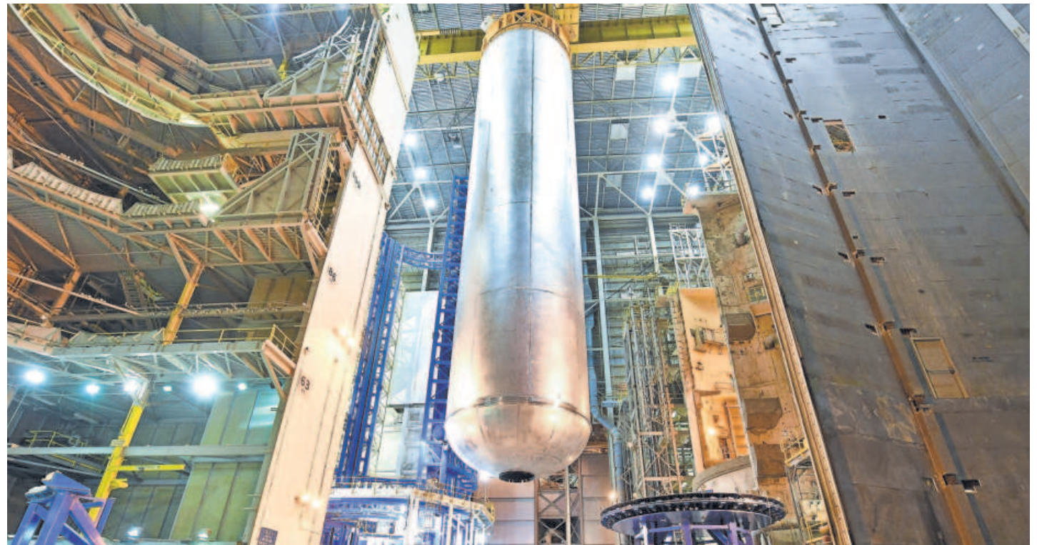
This 130-foot fuel tank, under construction in New Orleans, will go in the Space Launch System. STEVEN SEIPEL, NASA/MAF
