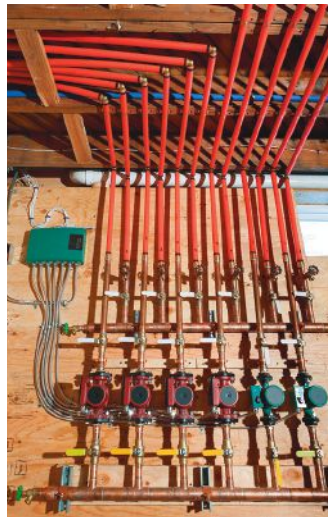
A zone heating system can help reduce peak energy consumption.
